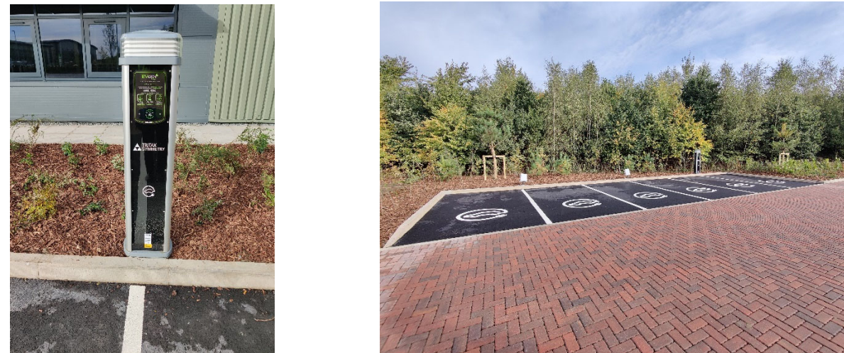
Fig 52. Examples of EV charging posts and bays within car park.
